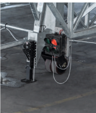
Signal and indicator lights
